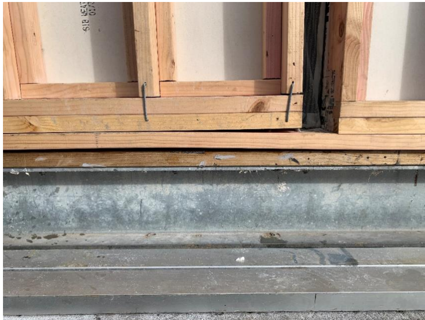
Figure 4: Deformation of the framing following the seismic lateral racking
